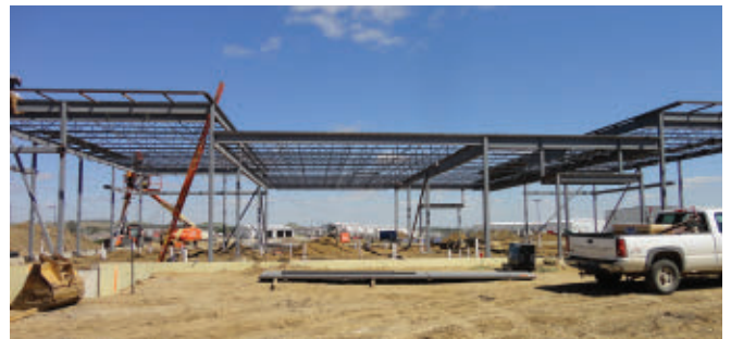
The Hub broke ground on its first location, a 7,800-square-foot travel center on seven acres in Dickinson, N.D. The store will feature 2,300 square feet of space devoted just to food. It’s set to open in October.
